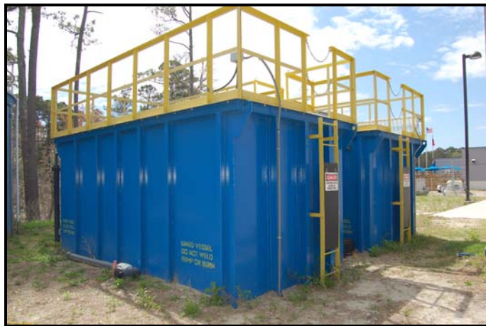
Tanks and Membrane Housing
